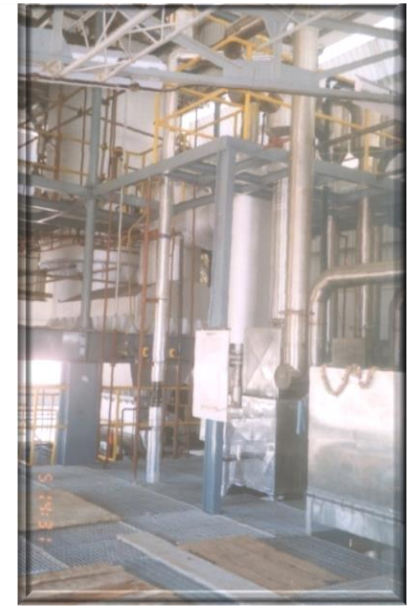
Gas Cleaning Unit
