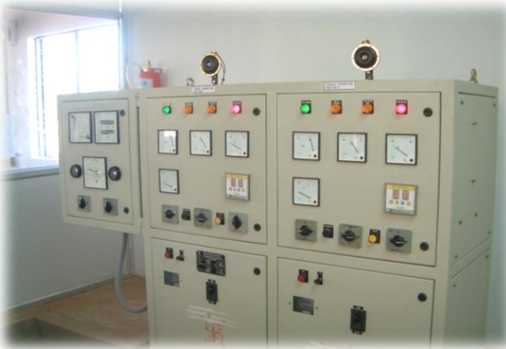
The gasification system and the power delivery panel
