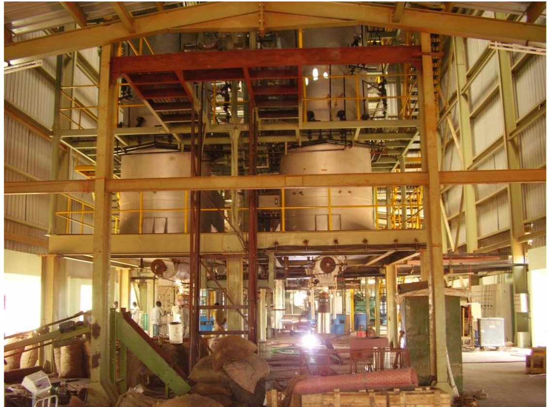
BMC GASIFIER PLANT(1700Kgph)
